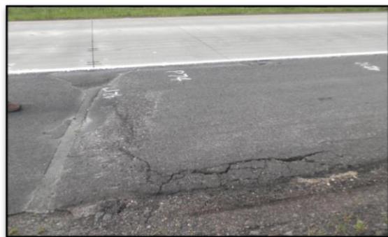
Figure C8.5. Block cracking Cell 13
