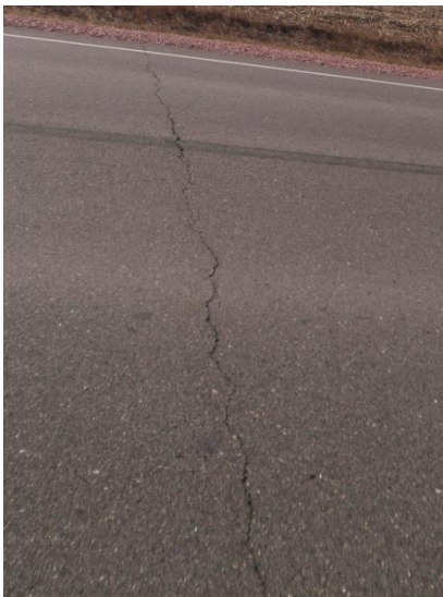
Figure B8.4. Low severity transverse crack (HMA 4% RAS)
