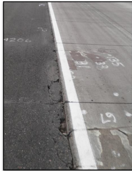
Figure C8.7. Alligator cracking Cell 14
