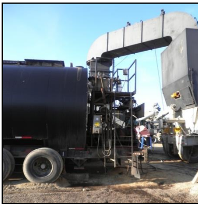
Figure E5.2. Evotherm® meter attachment to asphalt tank
