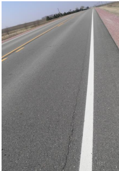
Figure B8.6. Longitudinal reflective cracking (HMA 0% RAS)
