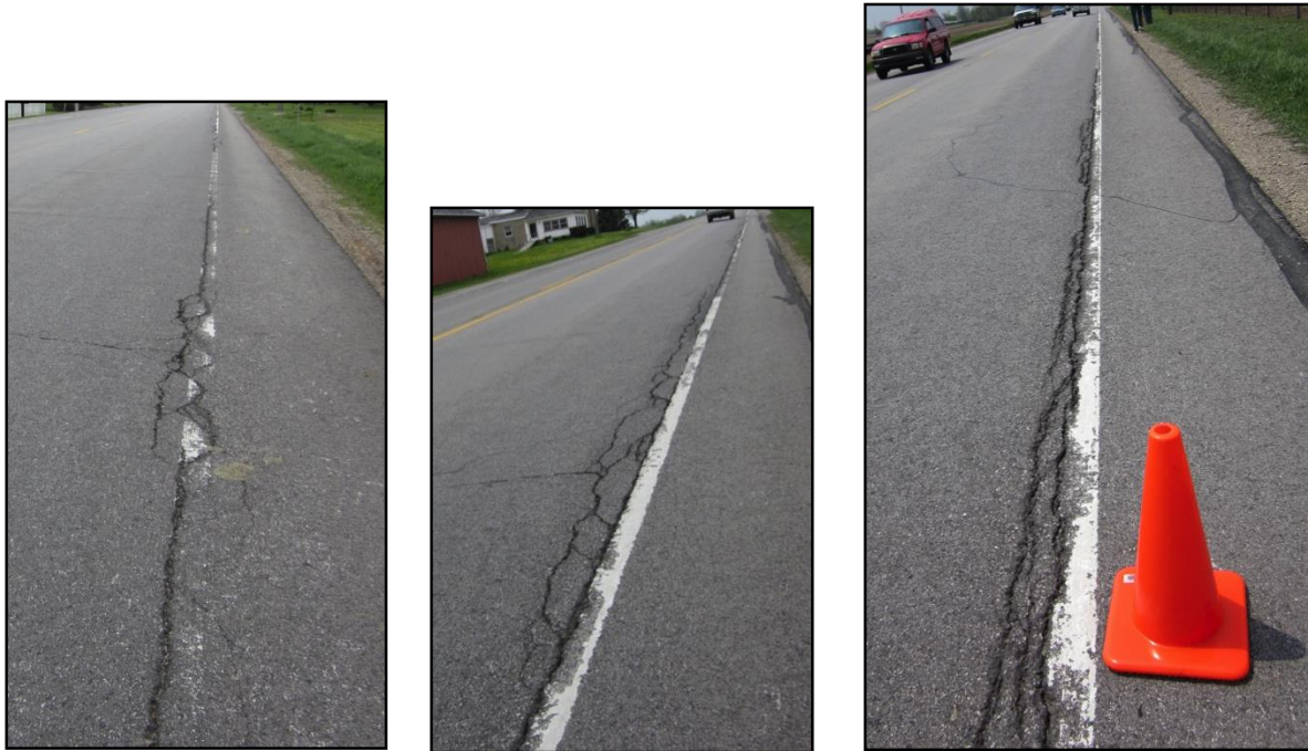
Figure D8.10. Longitudinal/block cracking near adjacent striping
