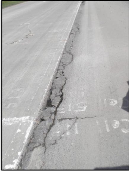
Figure C8.6. Alligator cracking Cell 13
