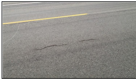
Figure D8.8 Fatigue cracking (WMA-RAS)
